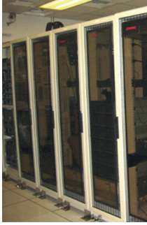
Computer server racks anchored to the floor
