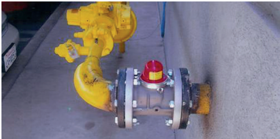
Seismic shutoff valve for natural gas line
