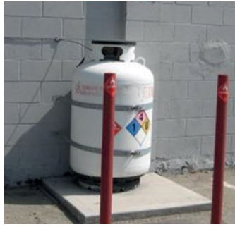
Flammable liquid tank strapped to wall
