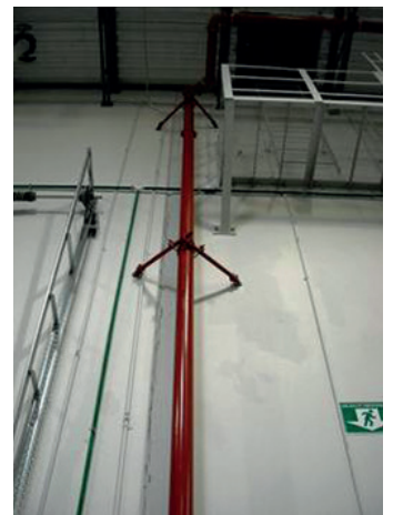
Sprinkler riser with sway bracing
